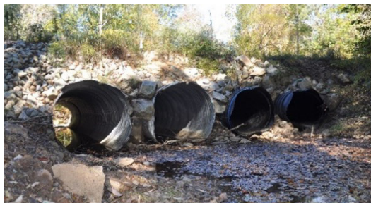
Undersized culverts at Gills Creek, SC. Credit: USFWS.
