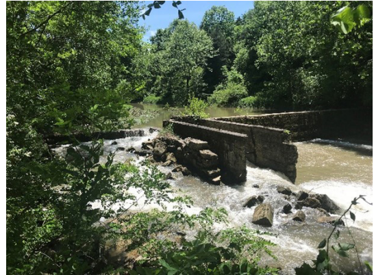
Little River Dam in Tazewell County, VA is slated to be removed with BIL funds. Credit: UFSWS.
