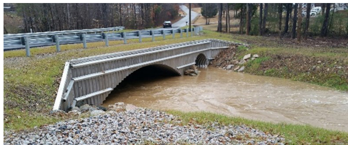
Gills Creek with a new culvert designed for fish passage. Credit: USFWS.
